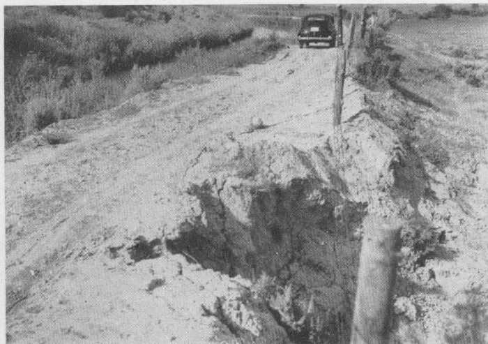
This canal bank is badly cracked as a result of seepage from the canal. The bank may fail at any time (Photo by C. W. Lauritzen)
